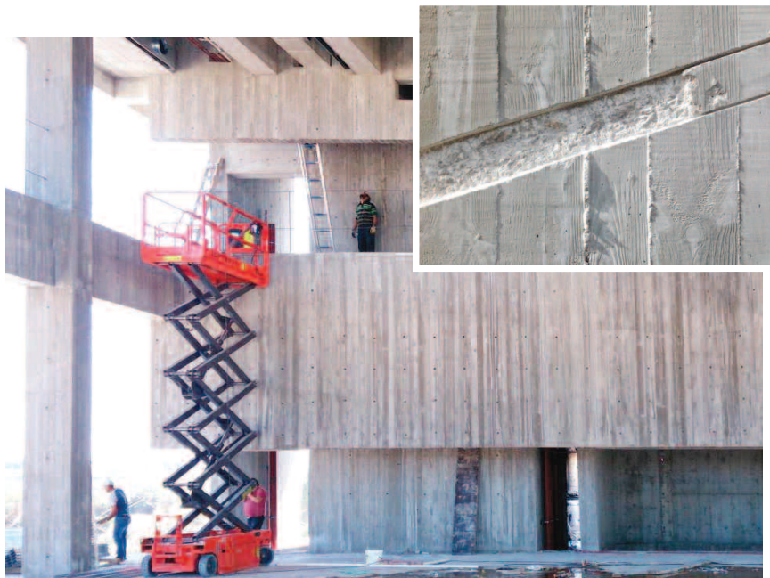
Photo 2. Wood formwork concrete – with imperfections of concrete and the traces of wood
