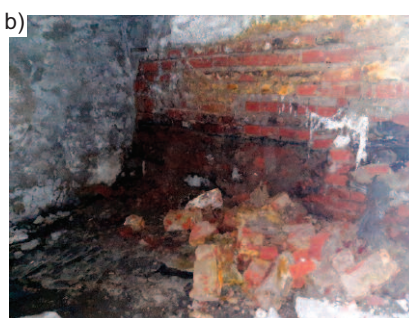
Photo 4. Damage to the walls of the underground part of the buildings: a) degradation of the wall bricks; b) delamination and collapsed part of the wall
