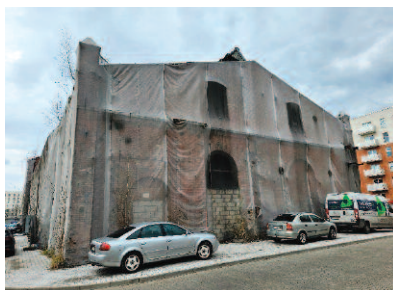
Photo 6. Front elevation with turrets proposed to be preserved as a historical witness
