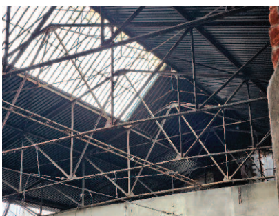
Photo 5. Trussed girders of the boiler room roof: extent of corrosion. March 2024 condition
