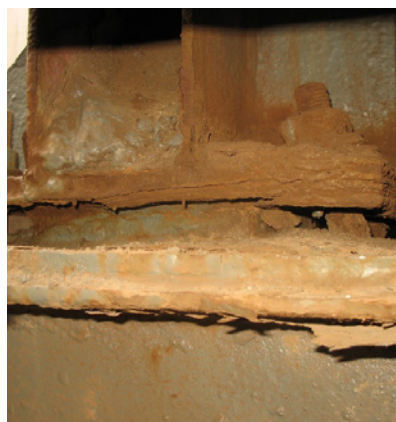
Photo 9. Corrosion and damage to the bolted connection of the gallery with the column
