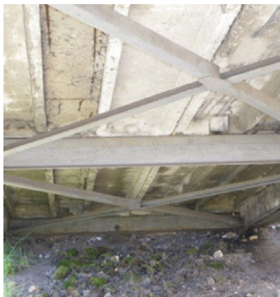
Photo 4. Blocked hinged movable supports
