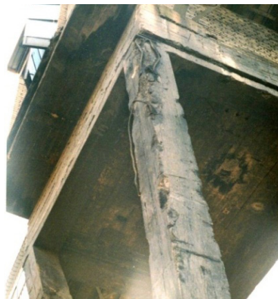
Photo 5. Advanced damage of tower columns
