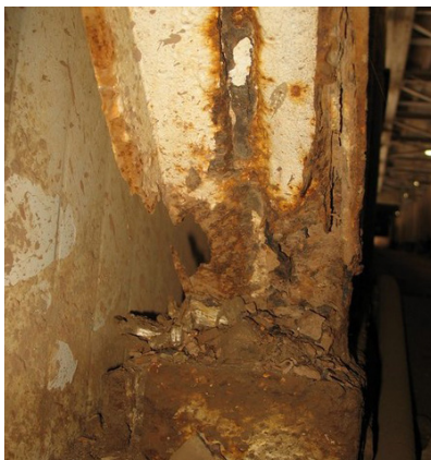
Photo 8. Pitting corrosion of the lower nodes – 90% cross-section loss, pre-failure condition
