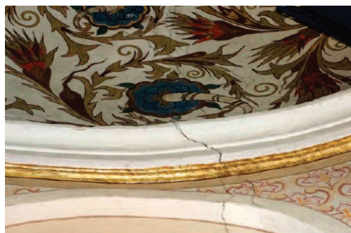
Photo 3. Example of damage to the part above the window
