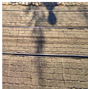
Photo 9. Concrete surface with the imprint of stone cubes, A. Wajda Street (11/2023)
