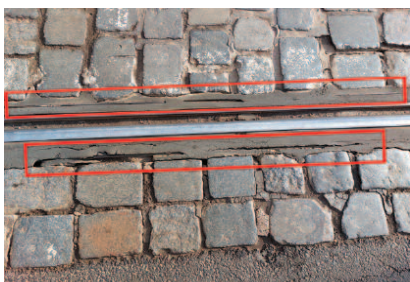
Photo 3. Tram track loaded with road traffic, loss of pouring mass, visible angle, Świdnicka Street on the section from Podwale Street to Kościuszki Square (12/2023)
