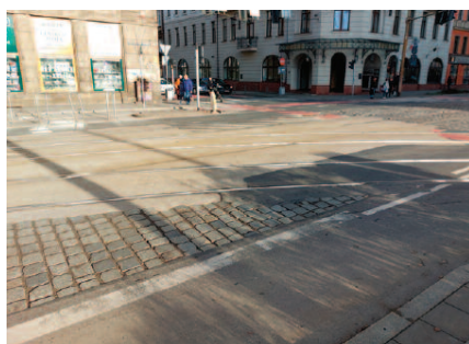
Photo 8. Visible extent of the concrete surface with the imprint of stone cubes in the area of the turnout, the turnout in J. Piłsudskiego Street, intersection with Stawowa Street (12/2023)
