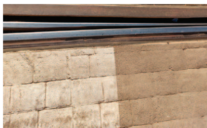
Photo 6. Tram tracks in the switch area, concrete surface with the imprint of stone cubes, turnout in the J. Piłsudskiego Street at the intersection with Stawowa Street (12/2023)
